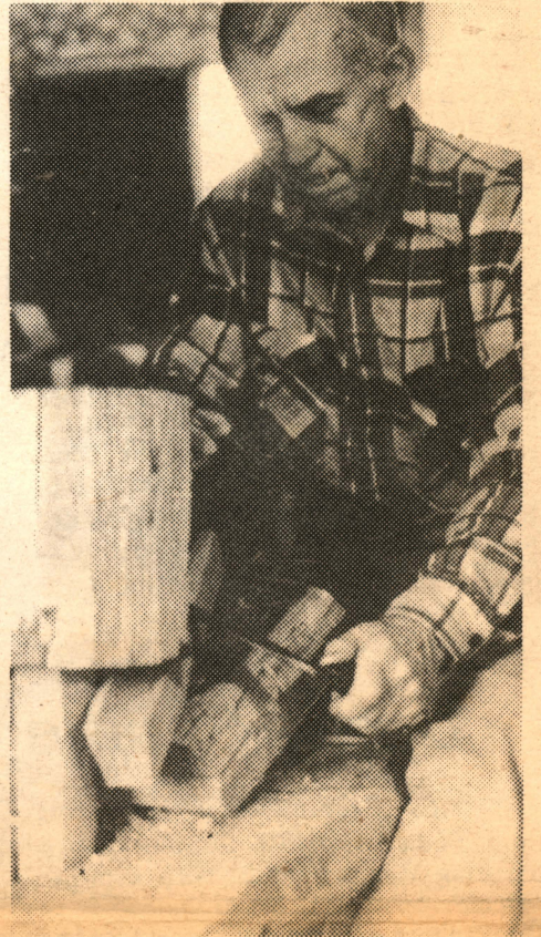
When the Wulster Barn is raised behind the Hopper-Goetschius House the beams will be held in place with trunnels made by Martin Knudsen of U.S.R. The volunteer carpenter says that hundreds of the wood pins used for fastening will be needed to secure the beams.
