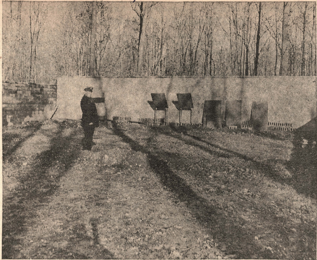
Ptl. George Bunning Jr. points to the armor plate target backings being set up in the almost-finished Waldwick firing range. Members of the police force and volunteers are building the structure.
